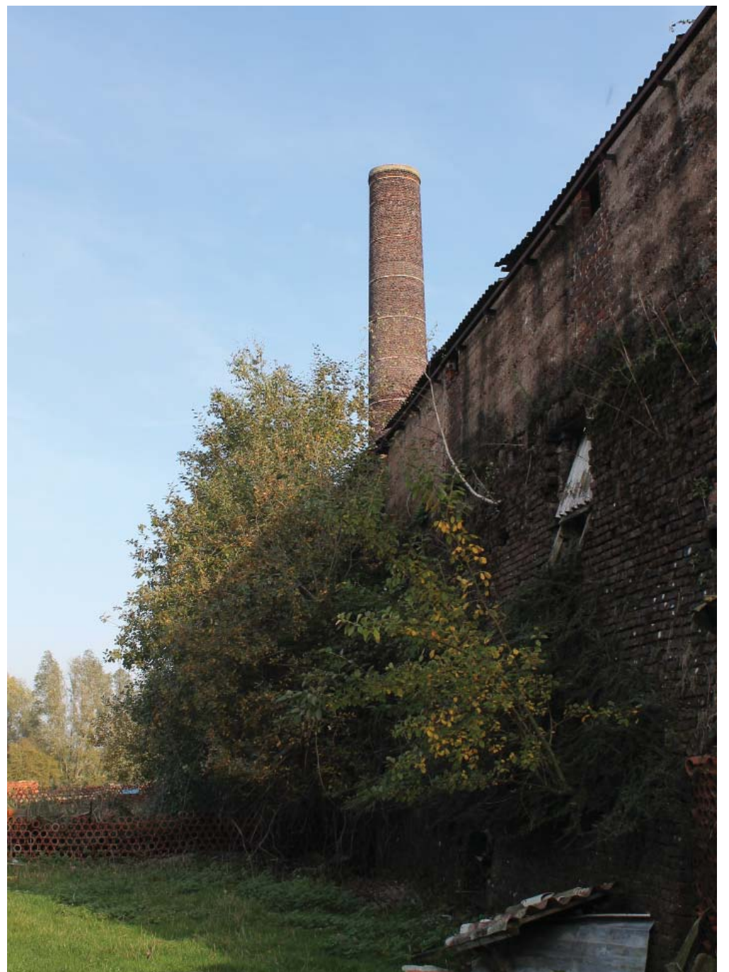
Larger plants growing out of the kiln walls
