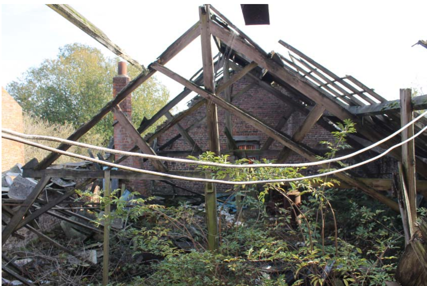
Missing roof of production building
