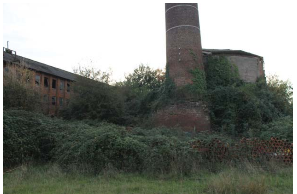
Vines growing up the chimney base with overgrown plants
