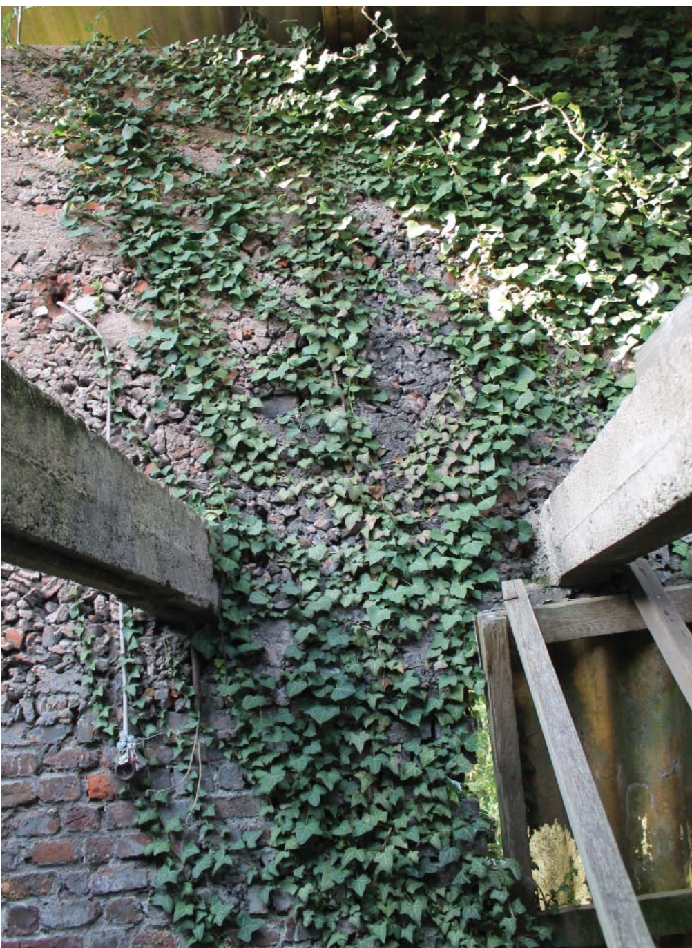
Vining plants growing on wall of kiln
