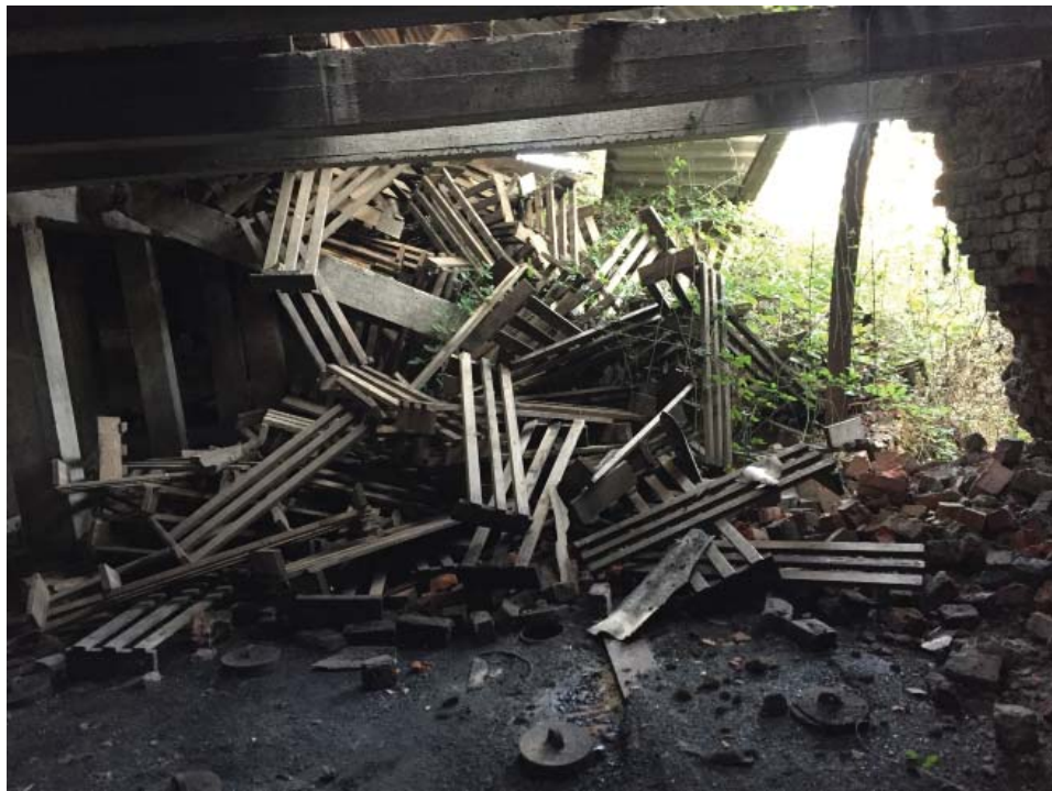
Collapsed wall of the kiln
