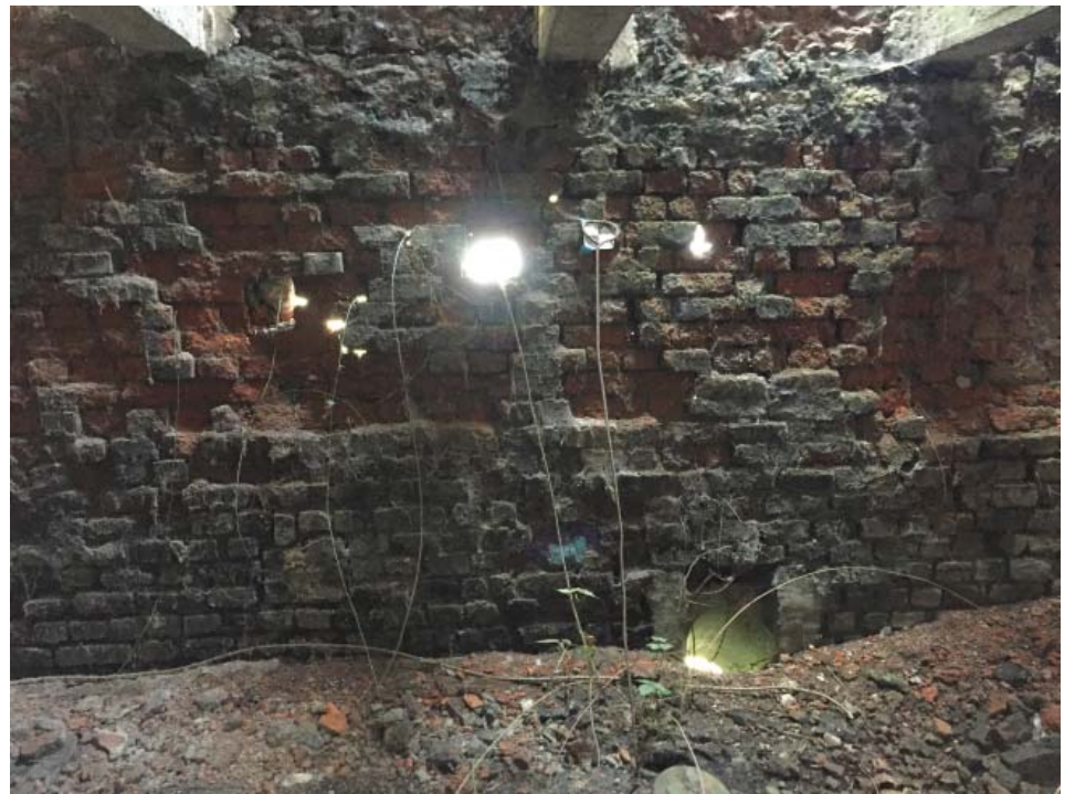
Material loss of the kiln walls
