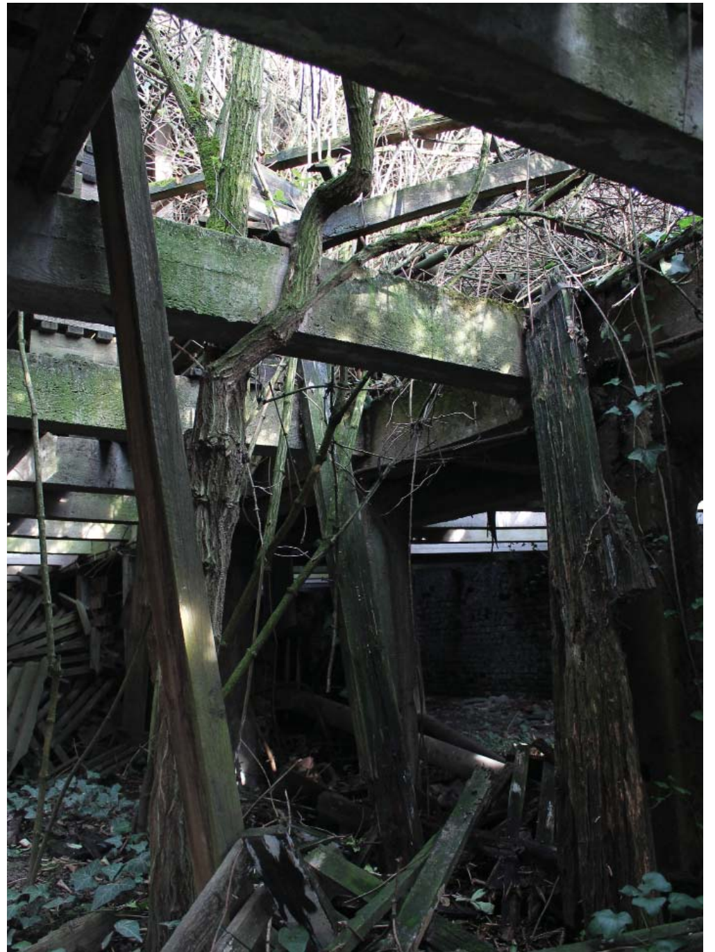
Tree growing around structural elements
