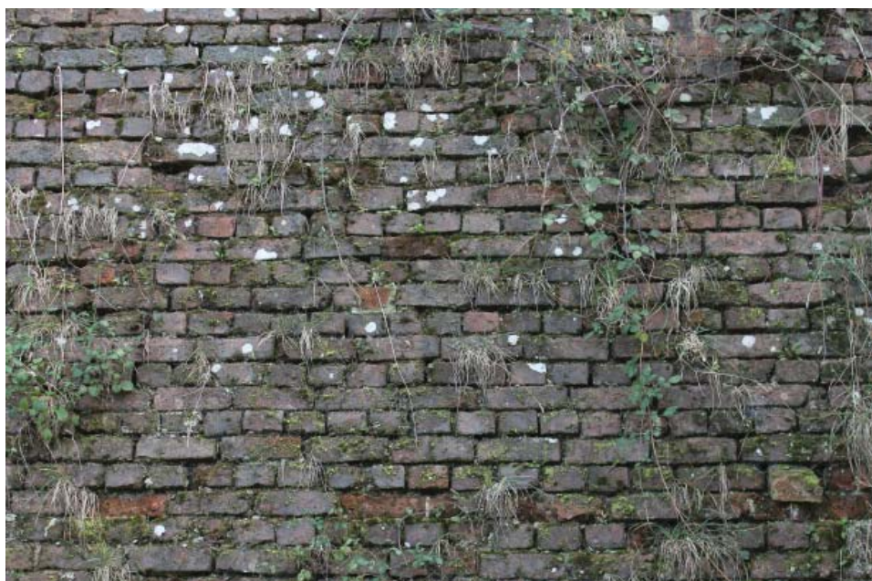
Biological growth on kiln walls
