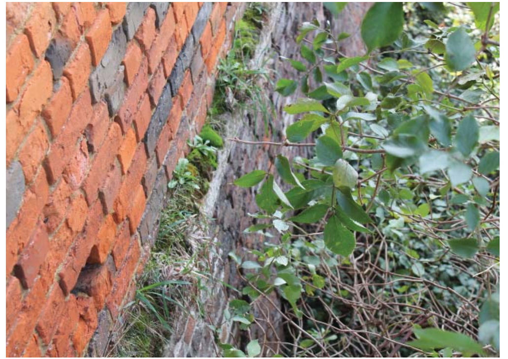
Biological growth growing in cracks of claytower
